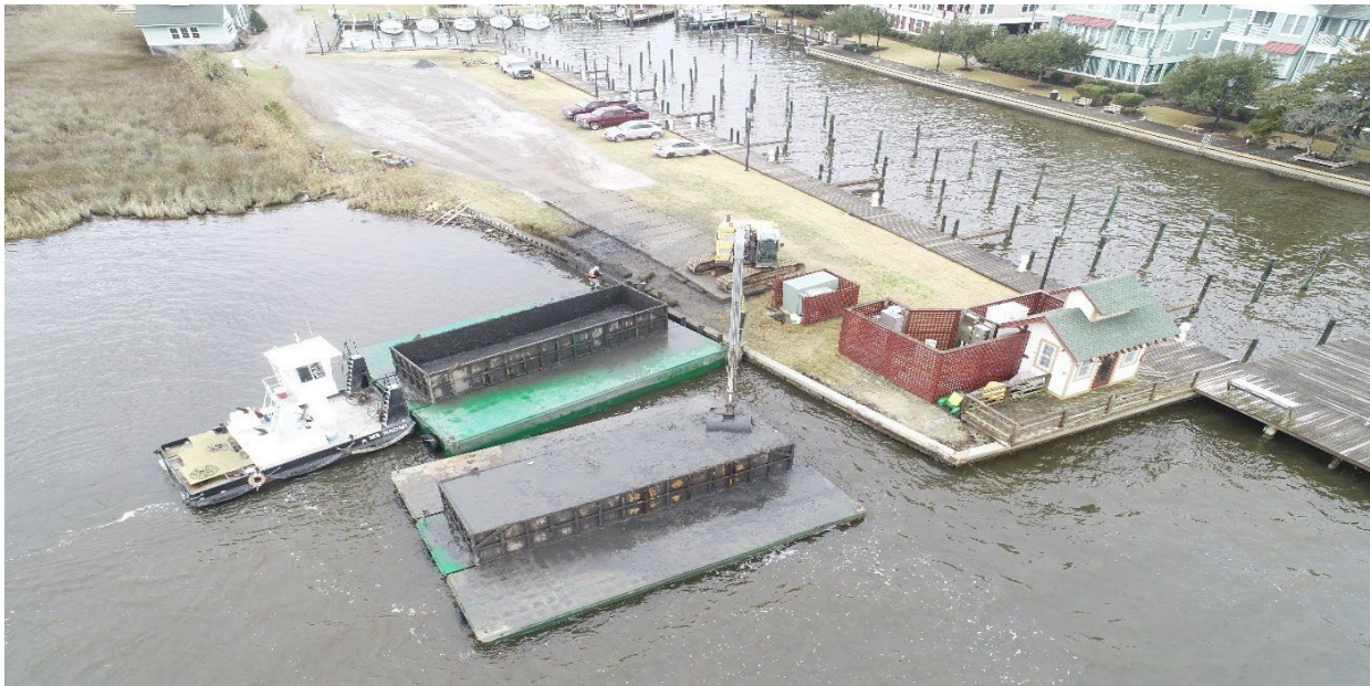
Dredge Material Transfer Station, Shallowbag Bay, NC. Source Credit: Dare County Grants and Waterways
